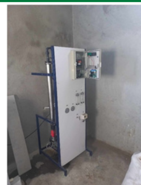
Figure 3. RO unit in the farm
